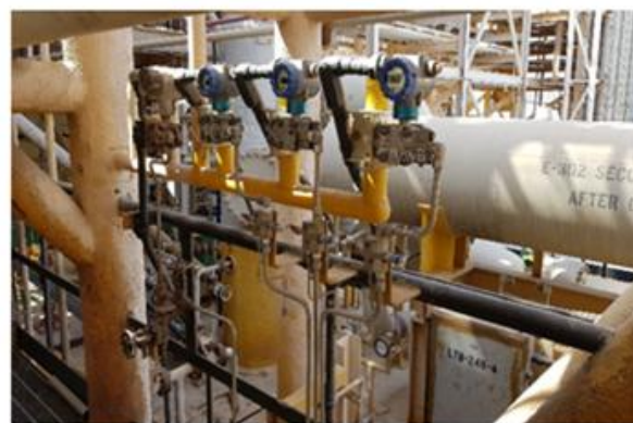
Fig. 9. Installed Transmitters for seal cavity pressure monitoring.
